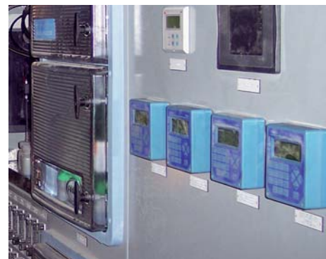
Four 770MAX instruments measure 16 channels of conductivity, dissolved oxygen and pH on sample panel by Waters Equipment.
