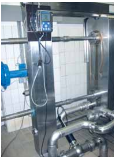
Fig. 2 Transmitter M 700 installed in conjunction with the InTrac 777.
